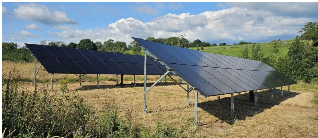
Above – Ground-mounted solar arrays
