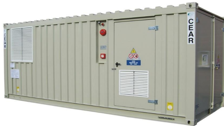
Above – Containerised HV / LV connection point
